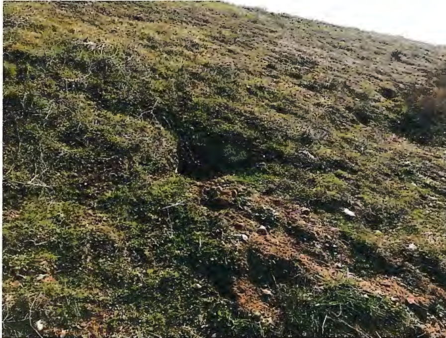
1. Large rodent hole discovered on the downstream face of the West Dike.
