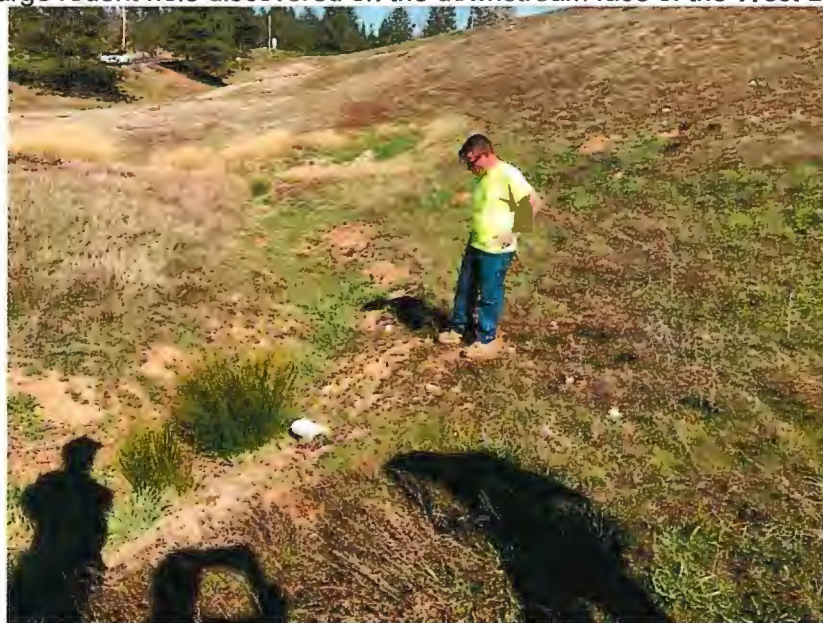
2. More rodent holes on the West Dike. Mr. Murphy inspecting the holes.
