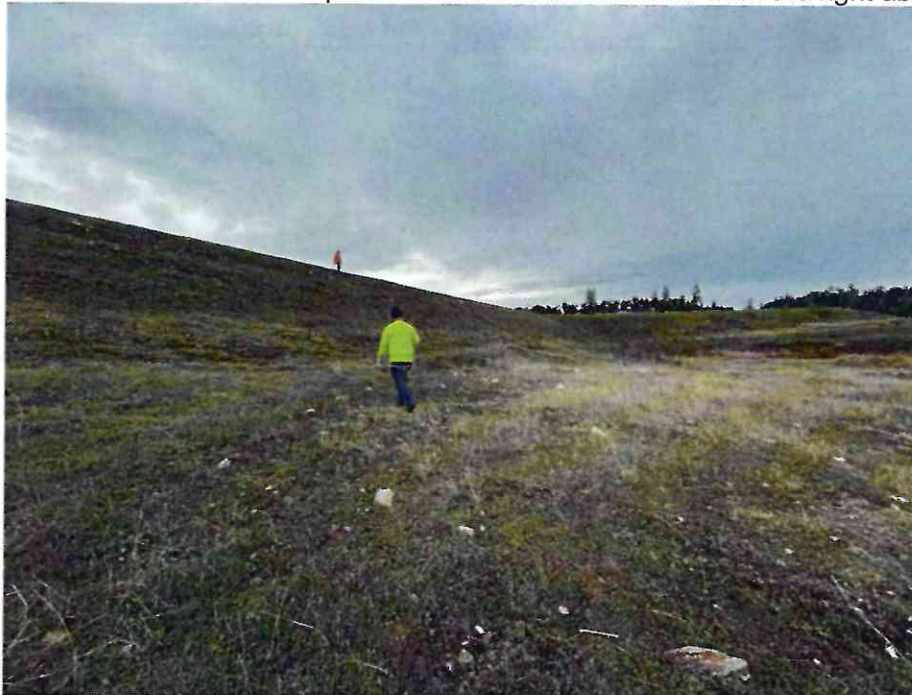
Photo 2: View of the downstream face of the West Dike from the right abutment.
